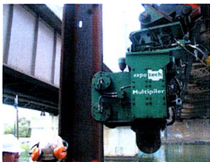
Multipiler in Melbourne driving LX25 sheet pile in 3 x 5m lengths to create 15m sheets.
