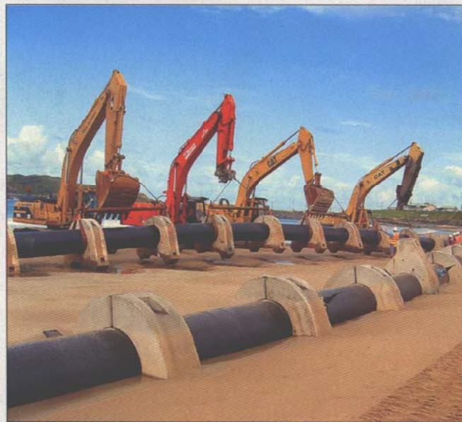
Four heavy lifting excavators were brought in to remove the two pipeline sections off Jetty Beach in Coffs Harbour.
